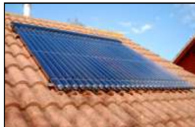
Solar thermal panel to heat water
